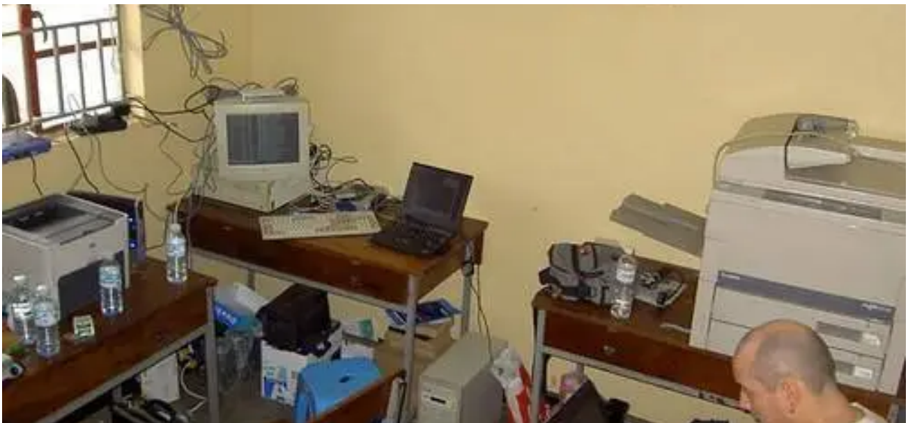
A small server room.
